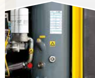
Element service vessel. Less than one hour needed to change the oil separator element.
