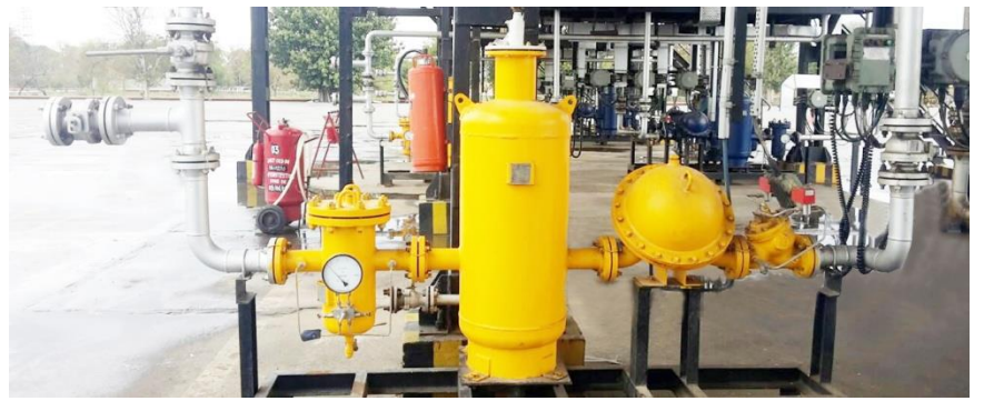
LC Metering installation – France
