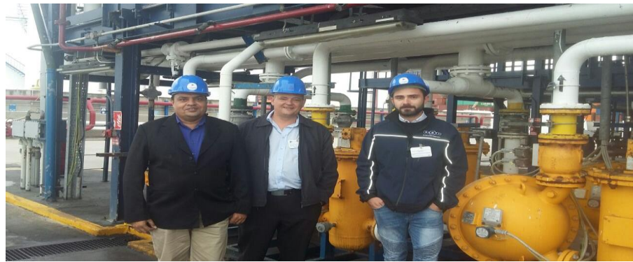
LC Metering installation – Florence Italy
