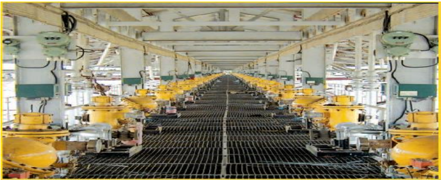
LC Metering installation – Florence Italy
