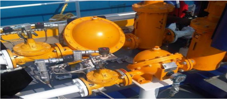
LC Metering installation – USA
